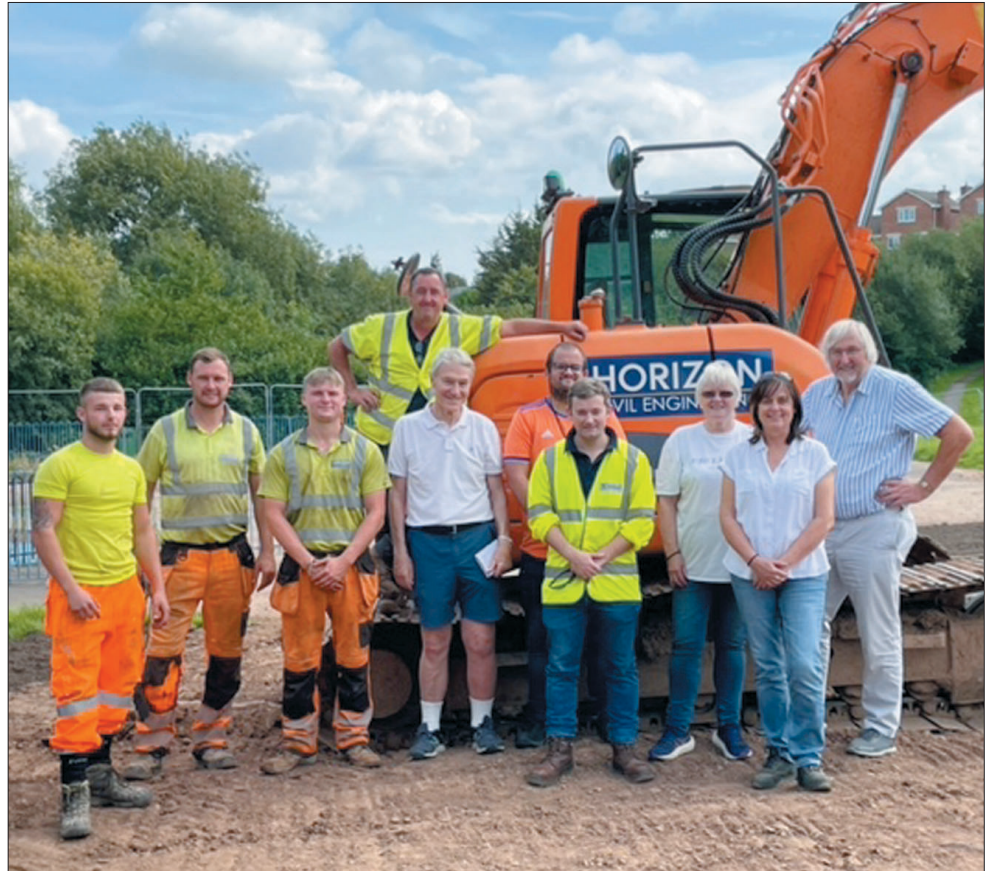
Helen Lloyd Jones with Council Officers and Horizon staff at the completion of the drainage work on Parc Radyr. Work on replacing the play equipment should start soon.
